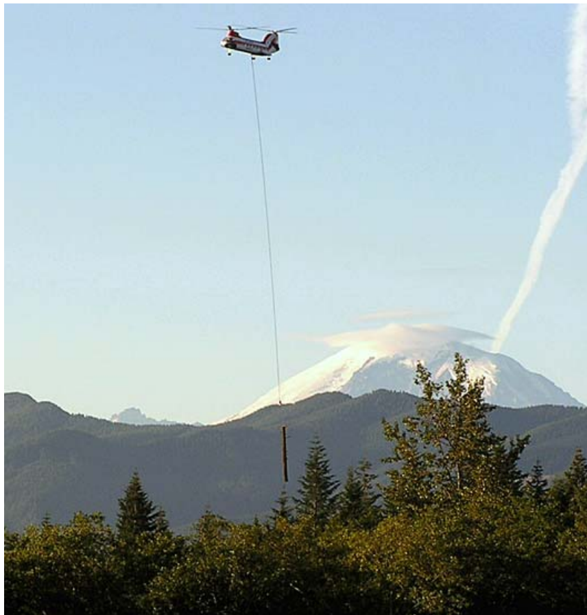
Just south of Mt. Rainier, BPA uses helicopters called air-cranes to remove logs cleared for the new Kangley-Echo Lake right of way. Logs are flown out of the Cedar River Watershed instead of being trucked to minimize environmental impacts to the area. Air-crane helicopters will also be used to transport and place transmission towers for the new line.
