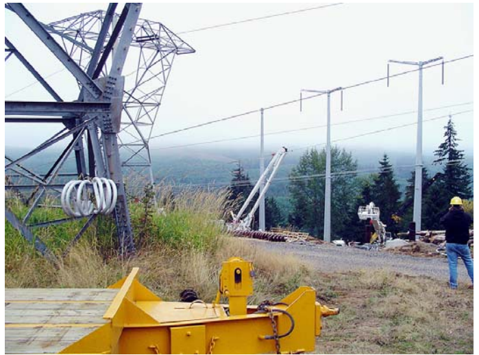
Snohomish and Chehalis Line crews setting off implosive line conductor splice on the SnoKing 500-kilovolt upgrade project.
