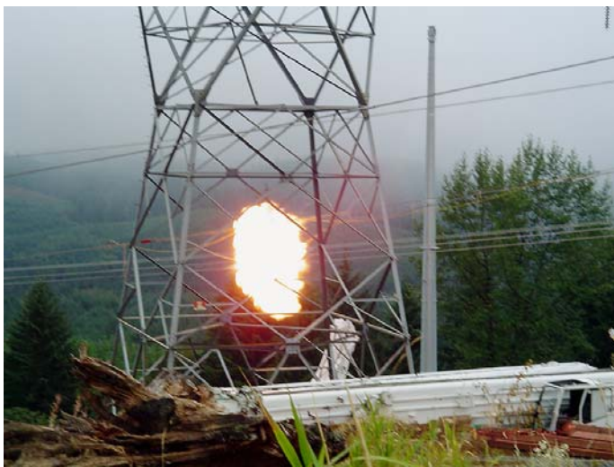
Snohomish and Chehalis Line crews setting new 25 thousand pound self-supporting tubular steel poles and completing implosive splices.
