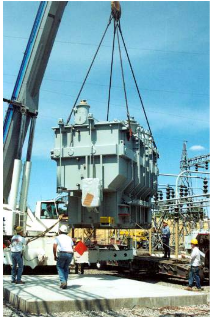
Bob Worrall's electrical services crew helps place the new transformer bank on the transformer pad at Walla Walla Substation.
