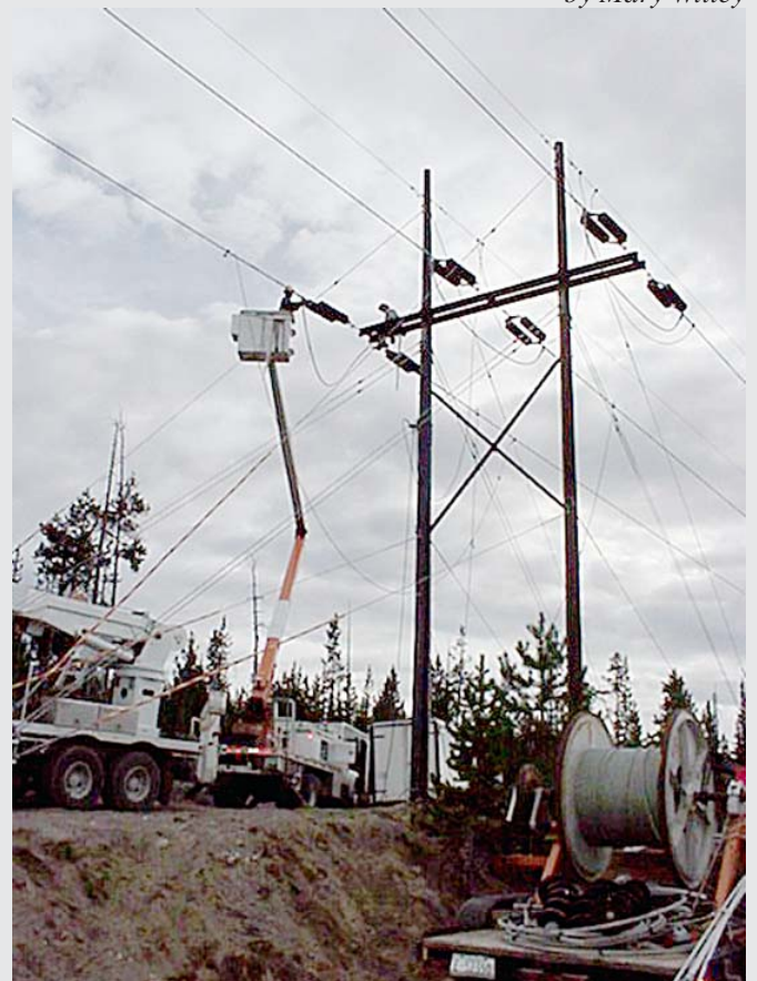
Idaho Linemen Travis Stanley (in the bucket), and Cole Bradbury (on the tower arm) are converting an existing A1 suspension structure to a dead end, in order to stabilize the conductors during ice unloading.
